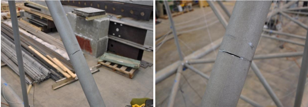
Figure 3.15: A third cut at back panel diagonal at bay 9 (damage case 1).
