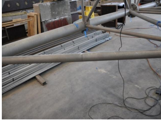
Figure 3.17: Multiple damage case: 90% cut at back panel diagonal at bay 9 and 90% cut at bottom panel diagonal at bay 5 (damage case 3).
