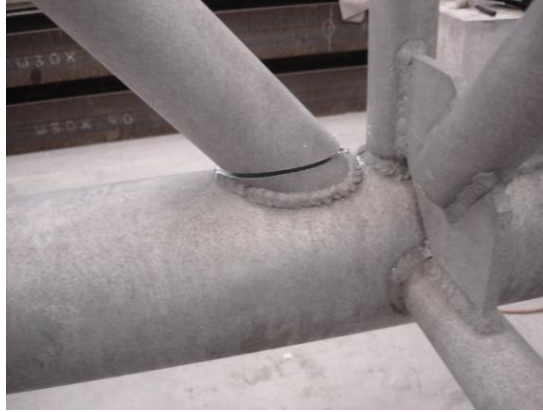
Figure 3.13: Damage case in Phase 1 of testing (a) Full Cut at bay 4 (Damage Case 5).
