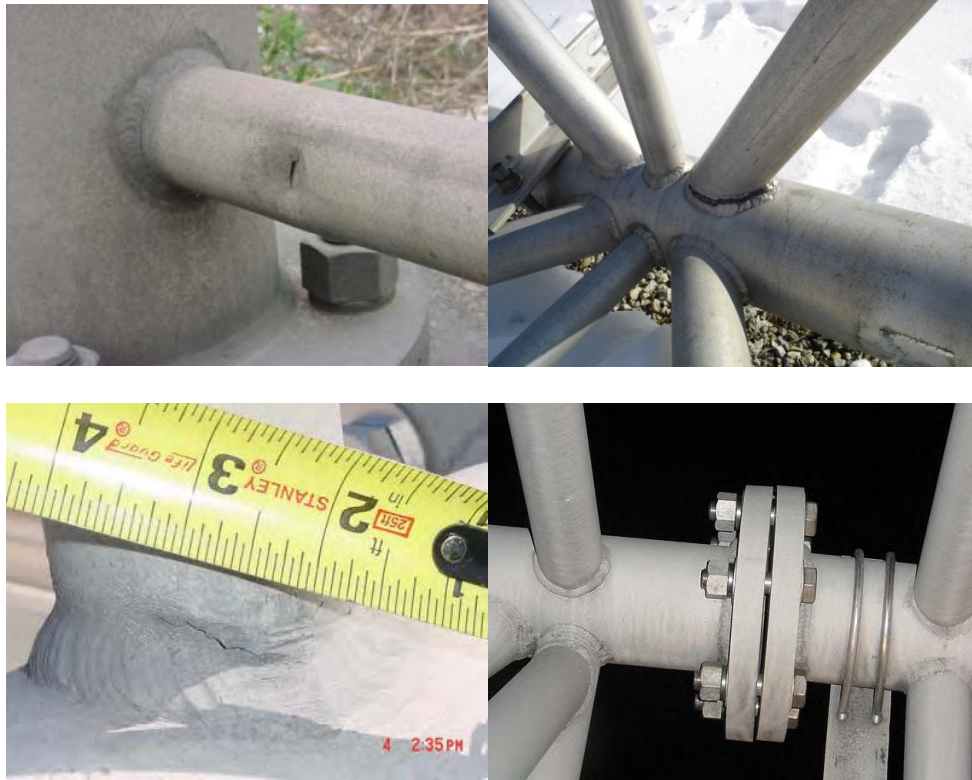
Figure 3.12: (a): Dent, tear, and weld crack in first strut on tower; (b): Weld crack in in-panel diagonal; (c): 1" long weld crack at lower chord; (d): Three loose fasteners that could not be tightened, Gap in chord splice.[46]
