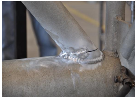
Figure 3.14: Damage case in Phase 1 of testing Half cut a bay 4 (Damage case 4).
